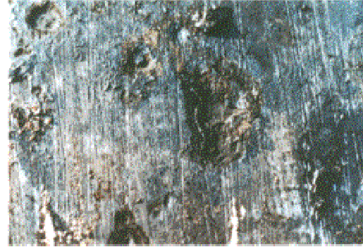
b. Corrosion in pit
